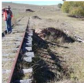
Probably deliberate removal of the embankment
