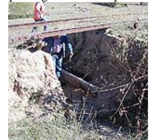
The worst culvert in an area where many sleepers were stolen.
