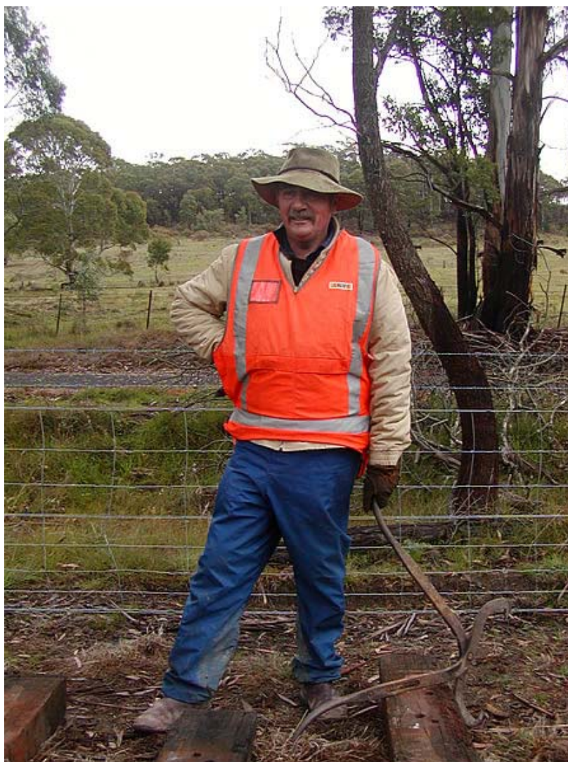
Graham pauses for a moment before lifting the replacement sleepers into place on the line.
