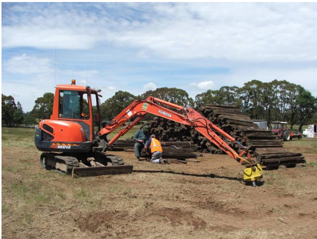
Ross Allen and Richard Webb sorting and bundling some of the thousands of sleepers OTHR purchased from ARTC. These sleepers were recently replaced by concrete sleepers on the main western line.
