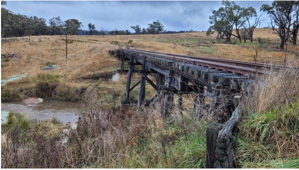
A recent photo of Snakes Valley Creek bridge at a recent inspection. Photo Michael Clark
