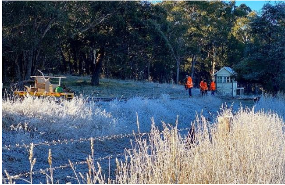
It was a cold and frosty start to work on the line by contractors CAM.
