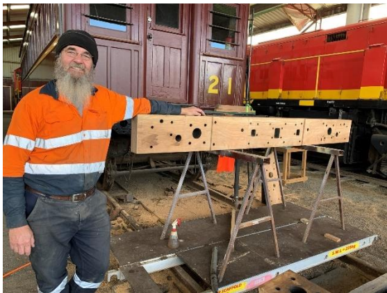
Michael Clark with a newly built headstock being refitted to the End Platform Carriage.
