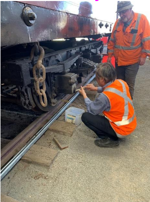
Some preliminary work underway for carriage inspections. Photo shows Tim Elderton and Dave LRW employee (standing) and OTHR working on the undercarriage.
