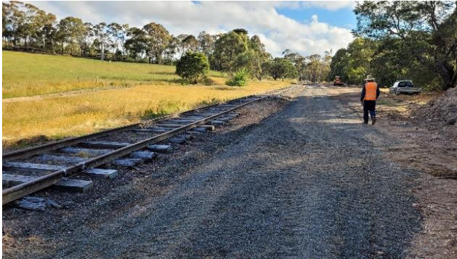
Base has been laid prior to the commencement of building the turnaround loop.
