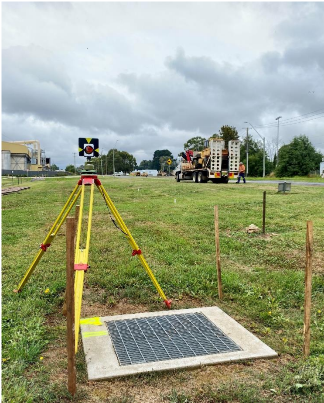
We had a surveyor on site every day - just to get the position and levels right
