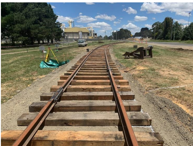
Sleepers and rail laid on to the east of Lowes Mount Road.
