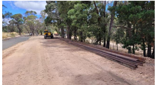
Rail for turn out at Hazelgrove, NSW.
