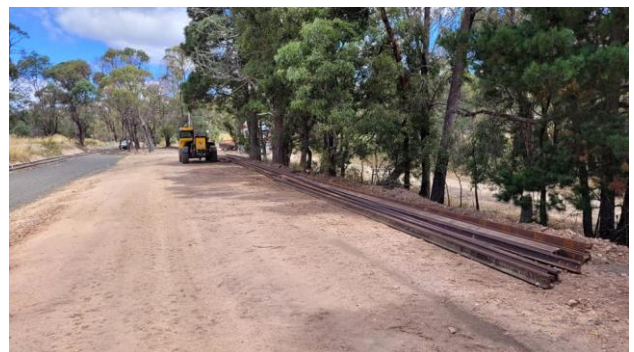
Rail for turn out at Hazelgrove, NSW.
