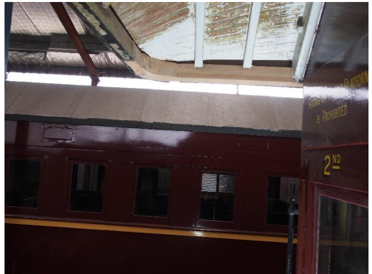
It was difficult to get a close up shot of the under-roof work of the end platform cars HL854. Flaking paint is evident and new timbers have replaced the very rotten existing.
