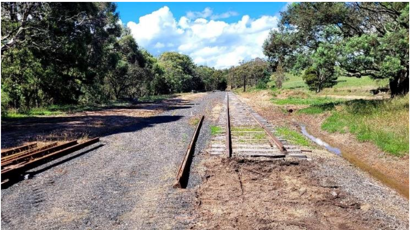
Resulting in a gap in the main line at the southern end of the station site.
