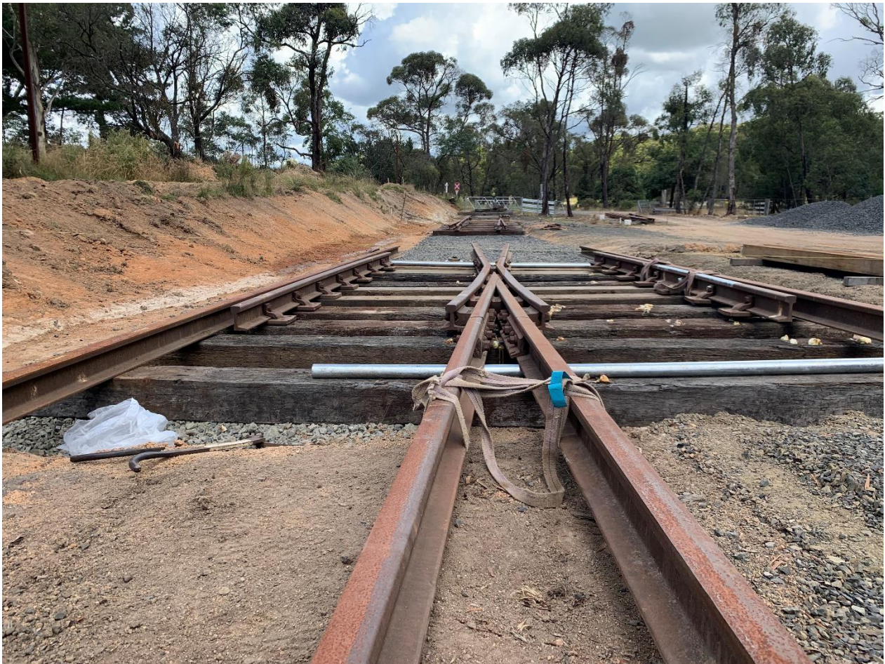
Southern crossing and check rails in place ready for "pinning down" this coming weekend
