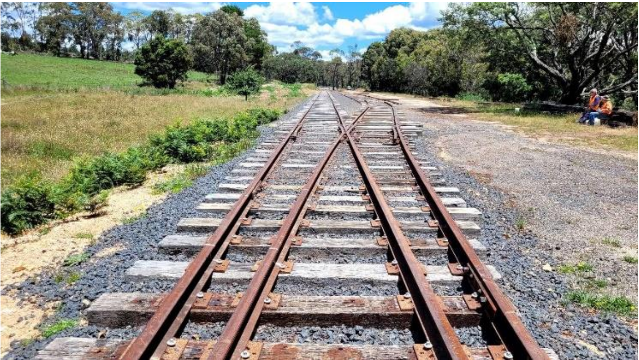
A view of the Northern Turnout and start of the loop line with rail snaking into the distance.
