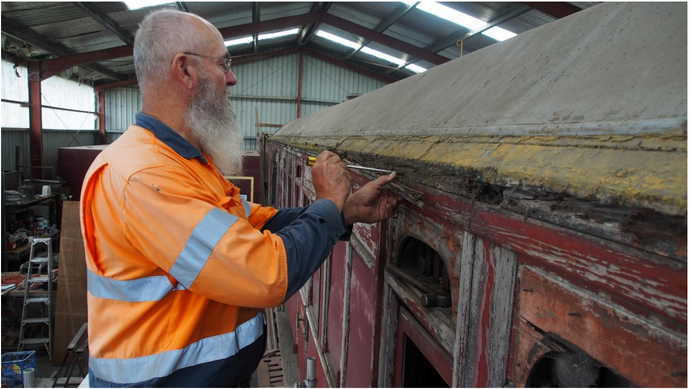
Checking out the timber under the guttering on HS36. Quite a bit of rot to deal with.
