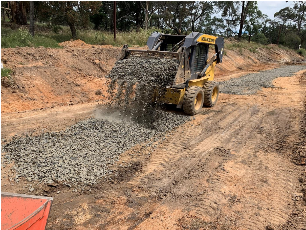
Adding bottom layer of ballast to the formation for the southern turnout
