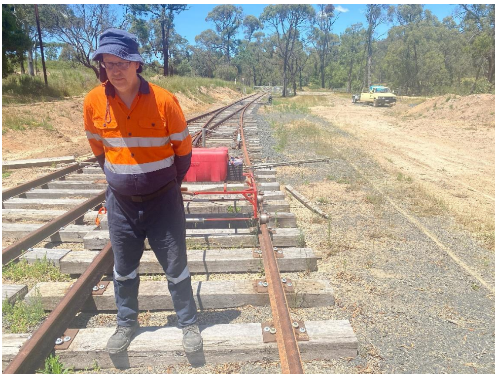
Trent Elliott moving the spray unit over the turnaround loop at Hazelgrove
