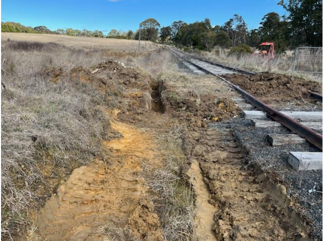
Near the 218.500 KM point work on the cess. A blocked pipe was removed. The job is not quite finished and you can see the water-logged soil in the foreground. Water that collects in the cess usually speeds up rotting of the sleepers
