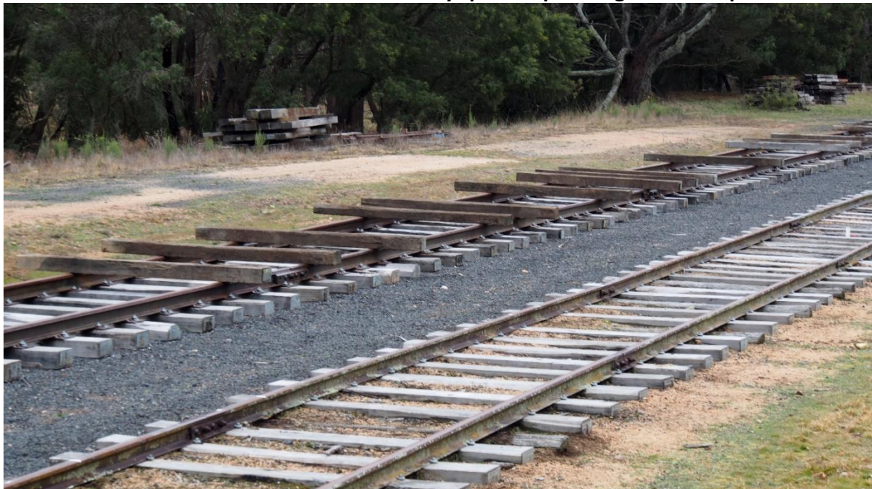
Sleepers stacked on the turnaround loop at Hazelgove. The 1 in 4 sleeper replacement in earlier work did not address all of the old and worn out sleepers.
