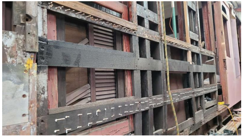
Lots of nail holes dowelled
